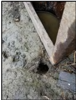
Figure 2. Leak near outlet caused by crayfish.
