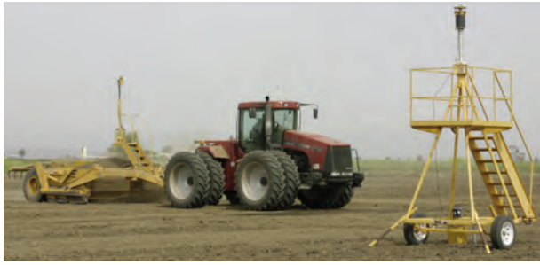
Figure 2. Typical scraper for leveling equipped with laser receiver that guides position of cutting blade. Signal is received from laser beam on stand in foreground. Scrapers may be equipped with single, dual or satellite guided receivers
